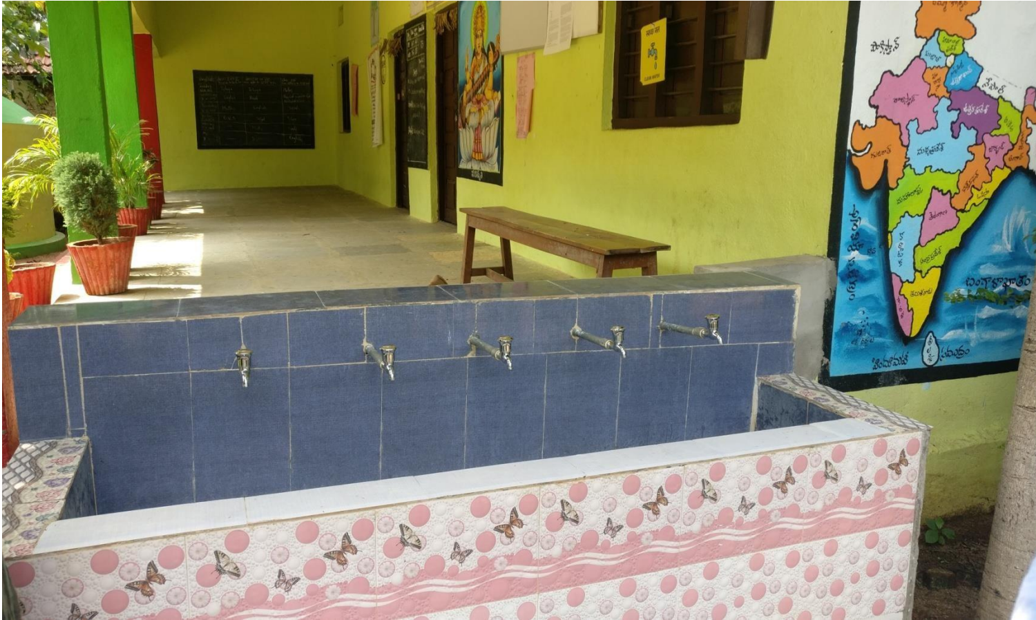
Drinking water facilities
